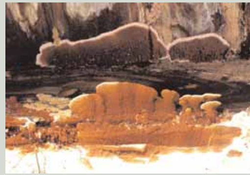
More damage can be caused to an old building by ill-advised dry rot treatments than by the original fungal attack itself
