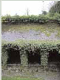
All plants growing against external walls should be clipped back regularly to avoid blocking gutters and concealing defects in the wall behind
