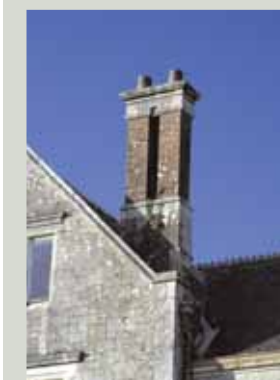
Chimney stacks are difficult to maintain as they are often the least accessible parts of the building but they are also the most exposed. Their condition can usually be monitored from ground level using binoculars
