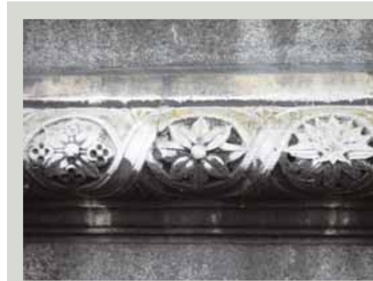
Some types of stone cannot be cleaned without unacceptable damage while other types may benefit from the removal of damaging soot deposits. It is important to get independent expert advice before undertaking a stone cleaning project
