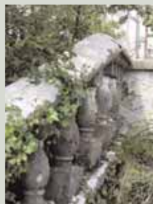
External features associated with a building such as walls and balustrades should be included in the maintenance programme
