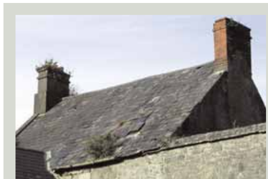
The roof provides the first line of defence for the interior of a building against the weather and it is essential it is well-maintained and kept in good repair
