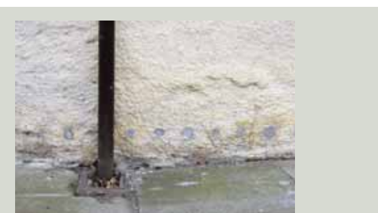
The drill holes associated with injecting a chemical DPC can be unsightly. A more effective method of dealing with the damp problem in this case would have been to reduce the level of the impermeable paving around the building and ensure that rainwater drains away from the base of the wall
