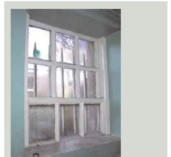
Condensation problems are best solved by reducing the moisture level of the air inside the building. While a dehumidifier may be useful for coping with the aftermath of an individual flood, the only successful long-term solution is to improve the levels of ventilation
