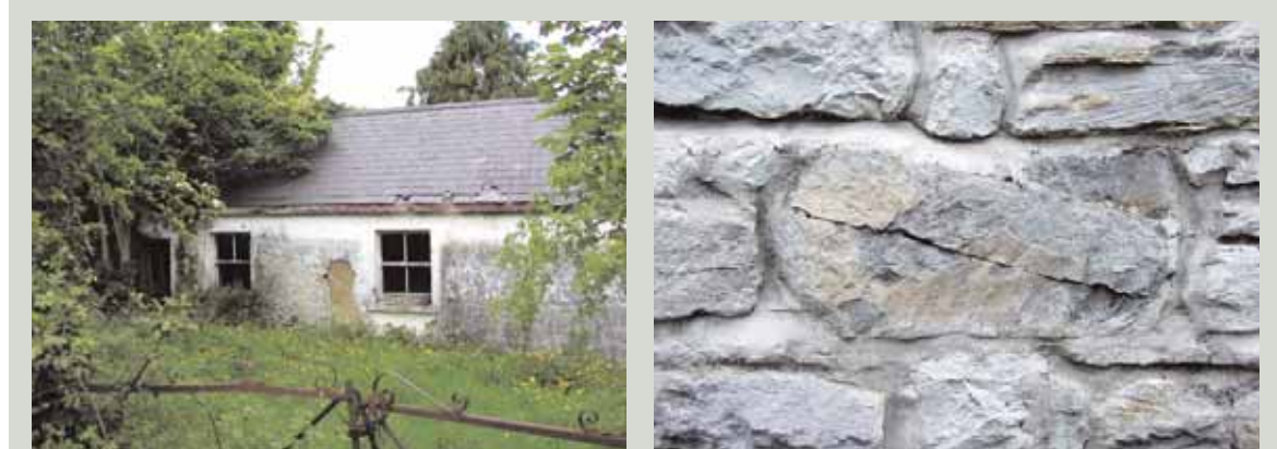
Traditionally-built buildings need to 'breathe', allowing the moisture absorbed during wet conditions to evaporate when the weather is dry. Inhibiting this process by letting trees and other plants to grow up close around a building or using the incorrect materials in repair can cause decay to set in
