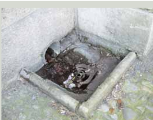
All gullies require inspection on a regular basis to ensure that litter or plant growth is not blocking the free flow of water
