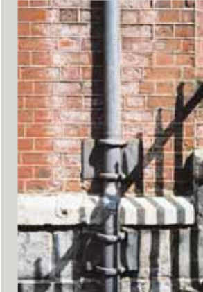
A white bloom of salts deposited on the surface of a wall, known as efflorescence, usually indicates saturation of the wall. In this case, the problem is almost certainly associated with the rainwater downpipe and needs immediate action to investigate the cause of the problem and to solve it
