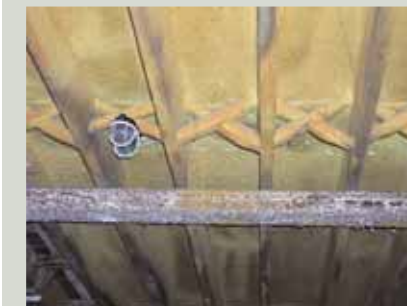
Spraying foams onto existing timbers, whether to increase thermal insulation or to enhance fire safety, is not advisable. Foams stop the natural ventilation of the timber structure, leaving it vulnerable to fungal attack. They are also difficult to remove
