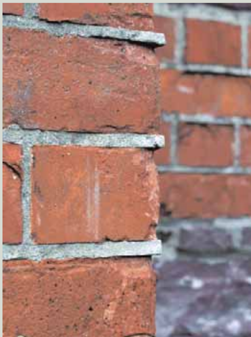
Cement-based mortars are hard and impermeable unlike the softer, more porous bricks seen here. Water moving through the wall cannot pass through the mortar, accumulates in the bricks and causes decay, particularly along the edges of the bricks. While the historic bricks decay, the cement mortar remains intact which is the opposite effect to what is wanted
