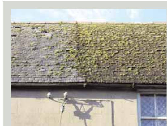
Moss growth is likely to take hold on more porous cladding materials such as clay or fibre cement tiles. It must be regularly removed from all roof types as it can force open joints between slates and tiles allowing water into the roof space
