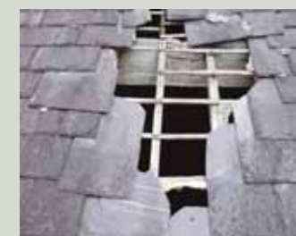
Slipped or missing slates must be attended to as a matter of urgency before damage is done by penetrating rainwater
