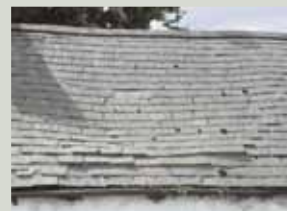
This roof is showing signs of sagging which probably indicates decay or damage of the structure beneath which must not be ignored
